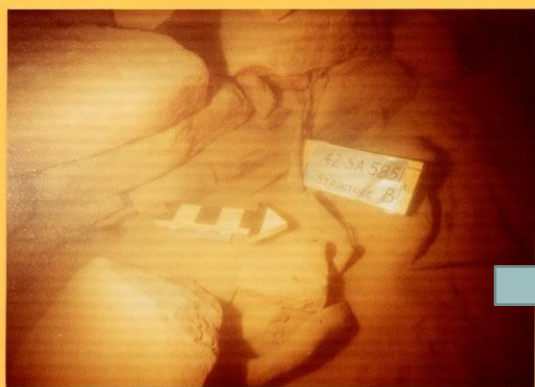
This small section of masonry wall from a submerged component of "Boll House" ruin was eventually stabilized by Larry Nordby. As far as we know, this represents the first time that an attempt has been made to stabilize an underwater masonry structure. Upon reexamination two months after stabilization, the epoxy grout seemed to be holding well. The site is located at a depth of 50', in a shallow sandstone alcove.
